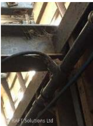
Figure 3. Example of changes in pipe diameter as pipework runs through a building
