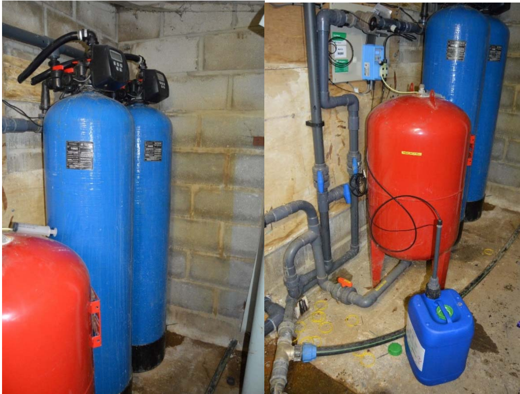
The new filtration and sanitisation system in place
