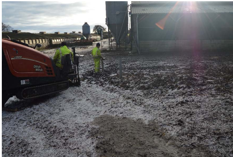
An operator with a detector at the front of the machine directs the borer
