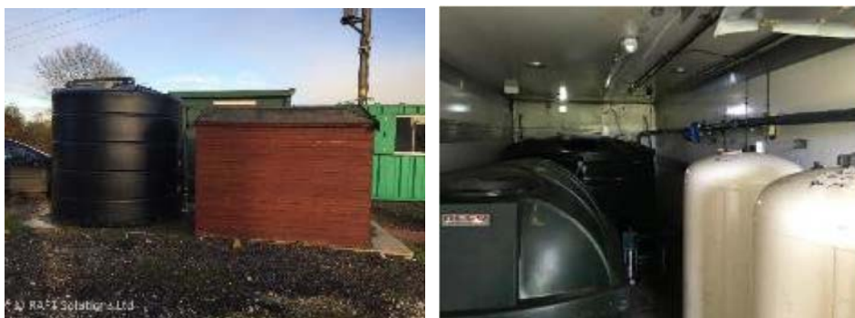
Figure 1. (left) and Figure 2. (right) Borehole and reception tanks
